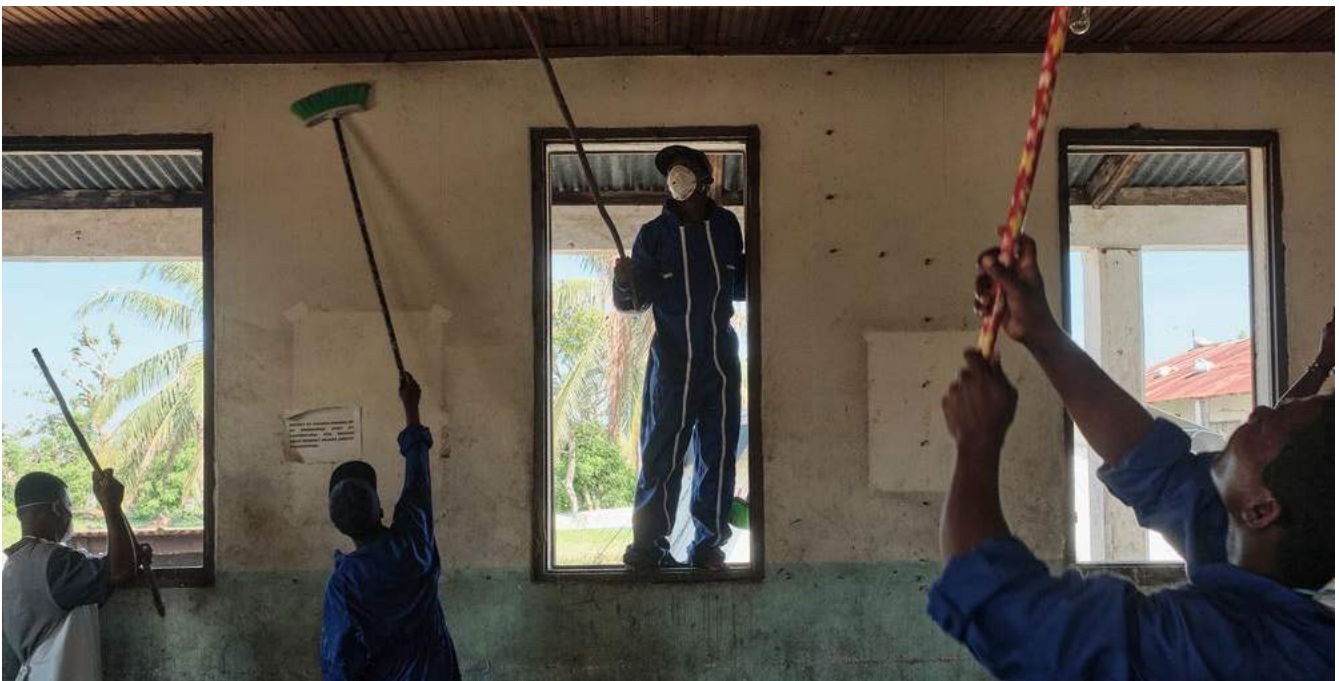
[MSB122807] Construction workers rehabilitate the hospital in Nosy Varika, Madagascar, after it was damaged by cyclones Batsirai and Emnati in February 2022. The storms were the latest in a series of shocks the country has faced in recent years. 1,2 iAko M. Randrianarivelo, March 2022.
