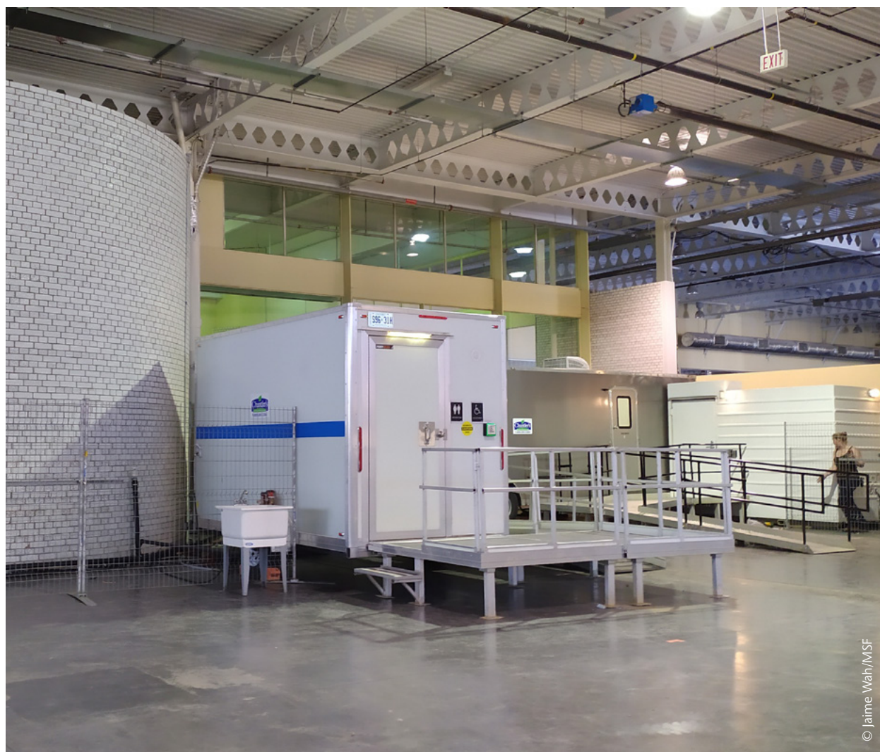
Accessible shower and toilet set up at the Better Living Centre, Toronto.
